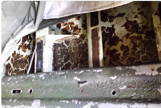
Mold due to moisture penetration and/or heat and moisture trapped under the cover.
