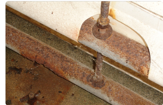
Corrosion can lead to structural weakness and failure.
